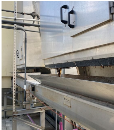
Backside of screens where screenings drop onto conveyor
