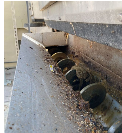
Auger in trough, note the wipe caught on the auger
