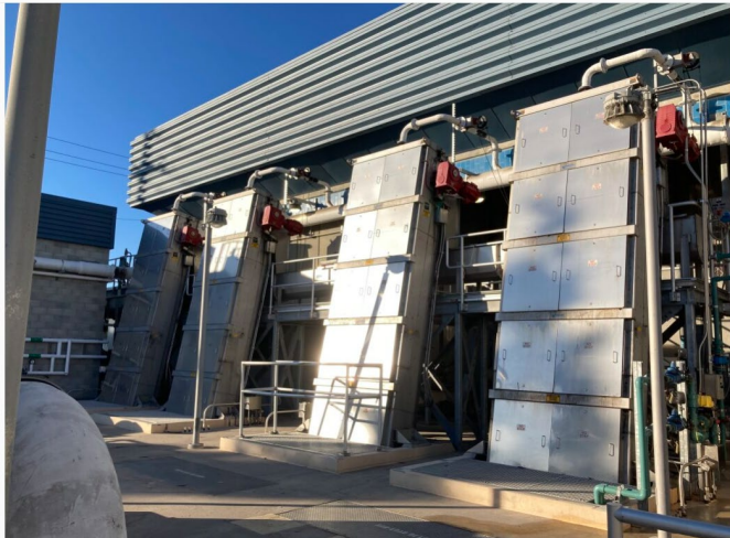
Four (4) screens with collection chute for screenings behind and gas extraction above.
