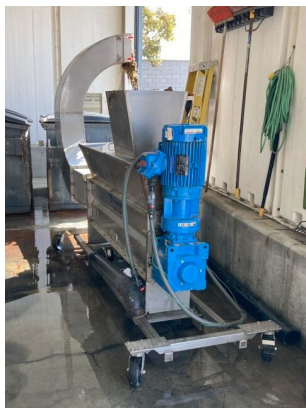
Washer , compactor unit – note the strung out material on exit chute
